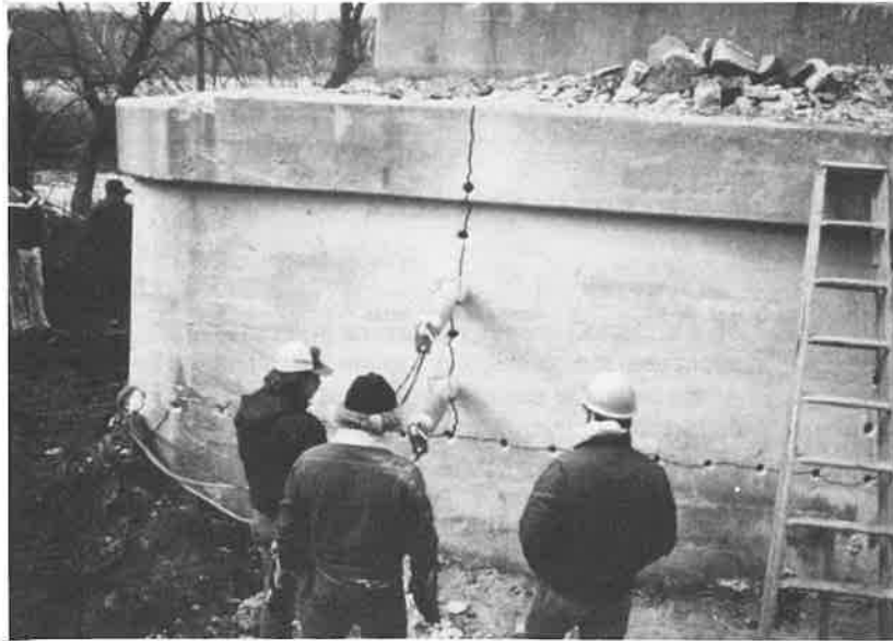
Bridge pier broken with two hydraulic splitters. Bottom section was saved for foundation of new pier.
