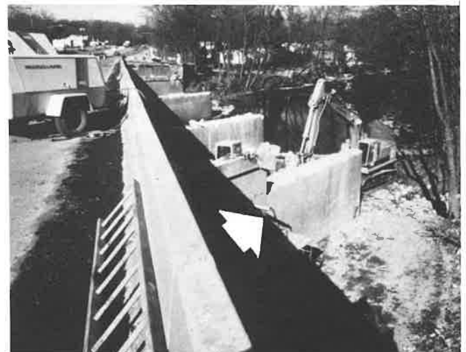
Several hydraulic splitters used to break bridge pier. This method allows the control of the length and direction of breaks.
