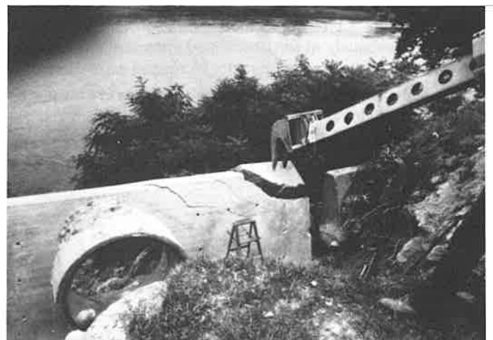
Broken pieces are easily pushed over with back hoe. This job was finished in hours rather than days.
