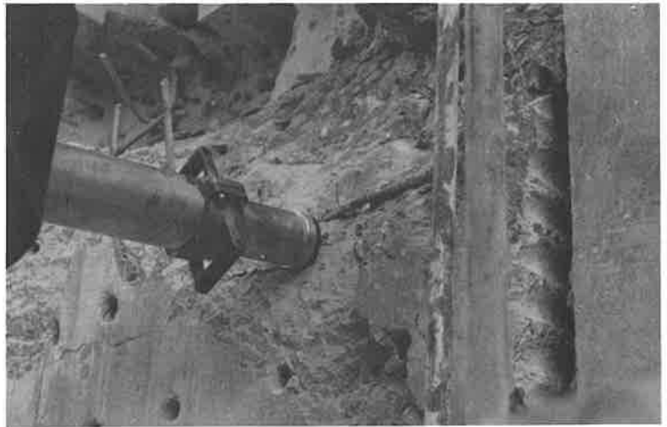
Start of an opening in a lock. (Note line drilled holes to right to create face.)
