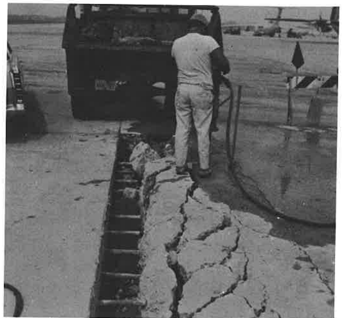
Example of controlled splitting. Note exposed rebar.
