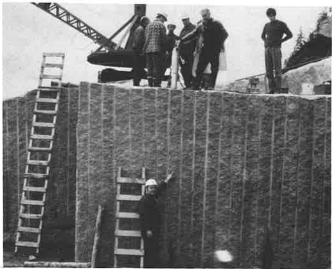
Three hydraulic splitters were used to split this huge section of granite. Size 30' x 12'. Break was made in 2 minutes.
