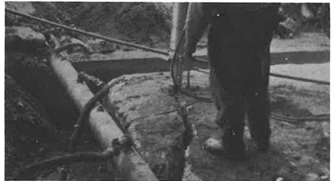
Floor slab cracks without damage to nearby equipment.
