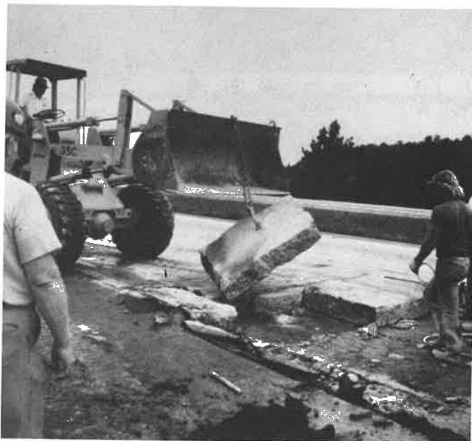
Large sections of concrete road is removed after split into sections with the hydraulic splitter.
