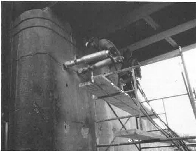
Top of bridge pier columns cut off with two hydraulic splitters. Remaining section to remain as base for new and expanded pier tops.
